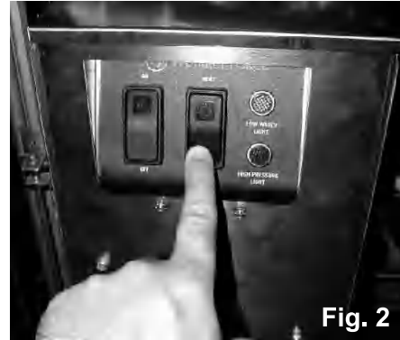
2. Energize heating circuit to pre-heat unit.
